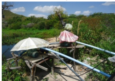
Moto bomba as margens do açude
